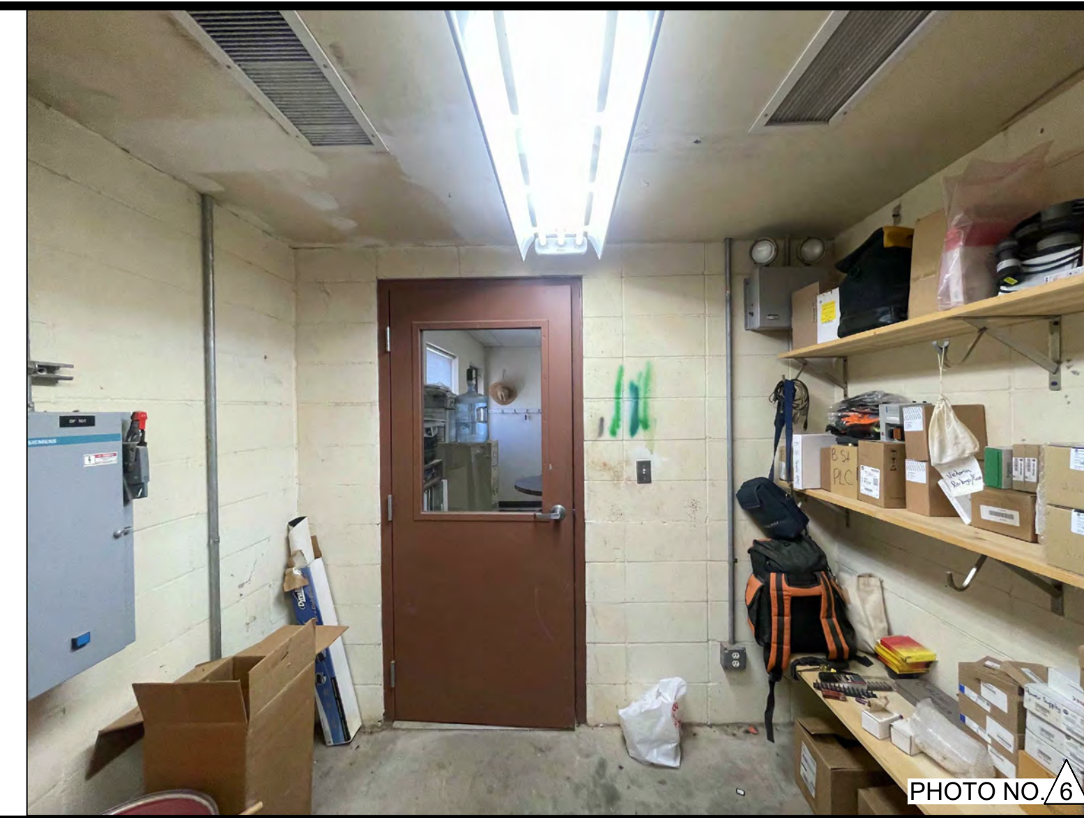
OPERATIONS BUILDING - PHOTO OF THE EAST WALL OF EXISTING ELECTRICAL ROOM.
