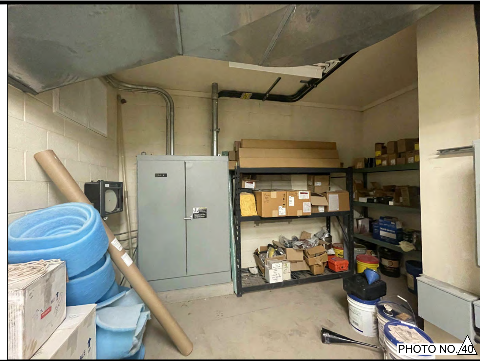
PHOTO OF THE WEST WALL OF EXISTING SLUDGE PUMP STATION UPPER FLOOR.
