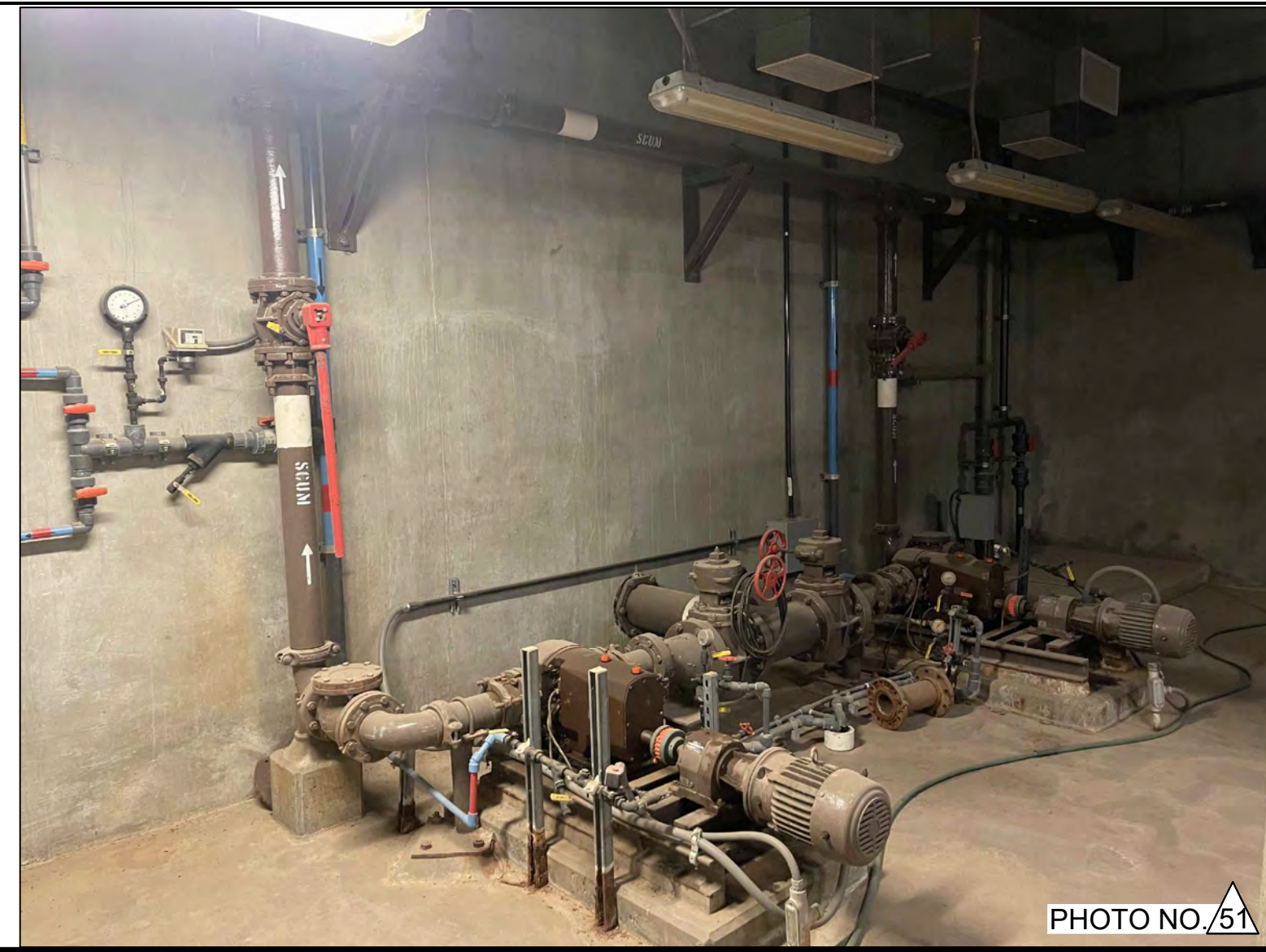
PHOTO OF THE SCUM PUMPS ON THE SOUTH WALL OF EXISTING SLUDGE PUMP STATION LOWER FLOOR.
