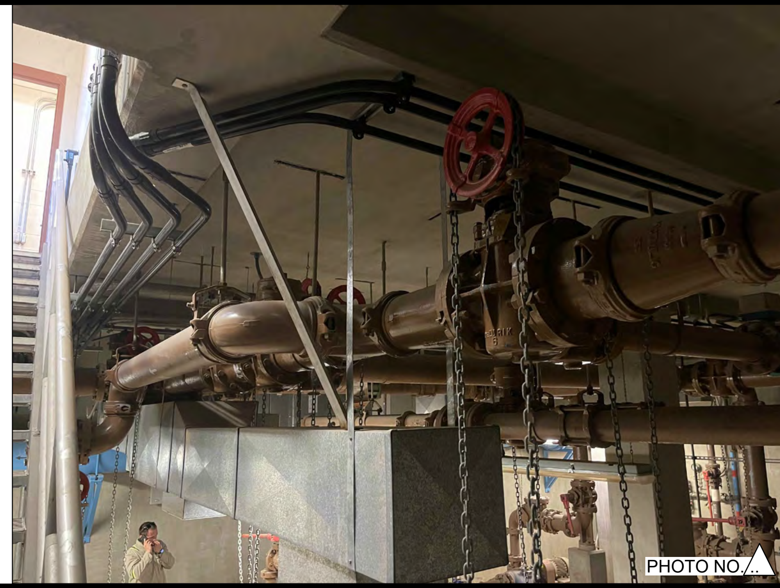
PHOTO OF THE OVERHEAD PIPELINES ON THE NORTHEAST SIDE OF EXISTING SLUDGE PUMP STATION LOWER FLOOR.
