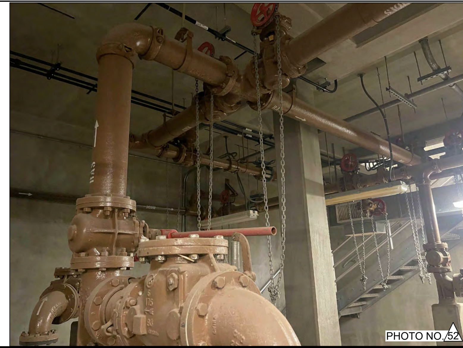
PHOTO OF THE OVERHEAD PIPELINES ON THE WEST SIDE OF EXISTING SLUDGE PUMP STATION LOWER FLOOR.
