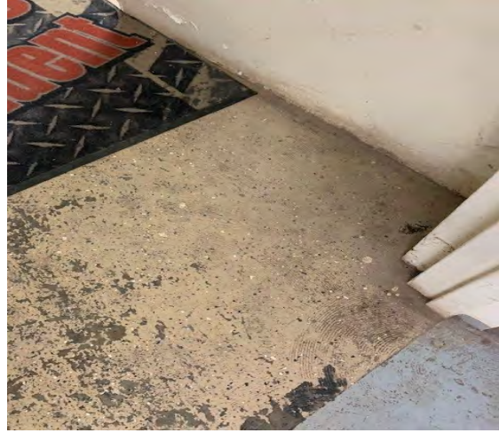
HM-8: Residual Floor Tile Mastic (ACM)
