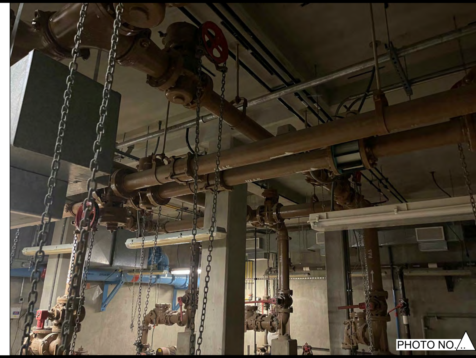
PHOTO OF THE OVERHEAD PIPELINES ON THE NORTHWEST SIDE OF EXISTING SLUDGE PUMP STATION LOWER FLOOR.
