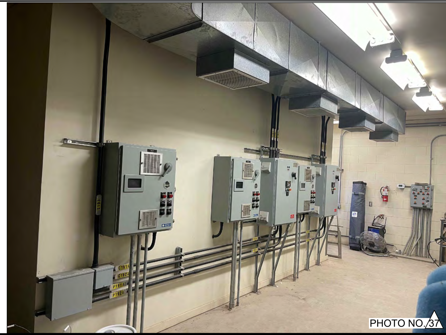
PHOTO OF THE NORTH WALL OF EXISTING SLUDGE PUMP STATION UPPER FLOOR.
