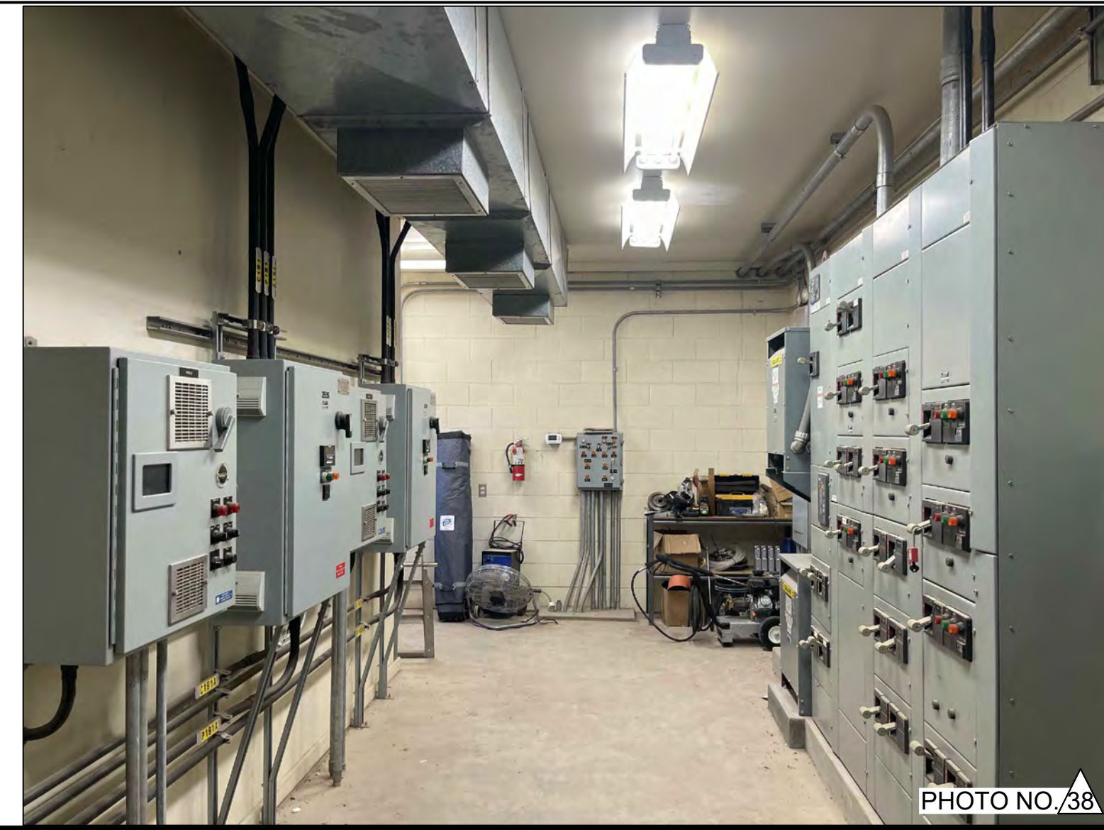
PHOTO OF THE EAST WALL OF EXISTING SLUDGE PUMP STATION UPPER FLOOR.
