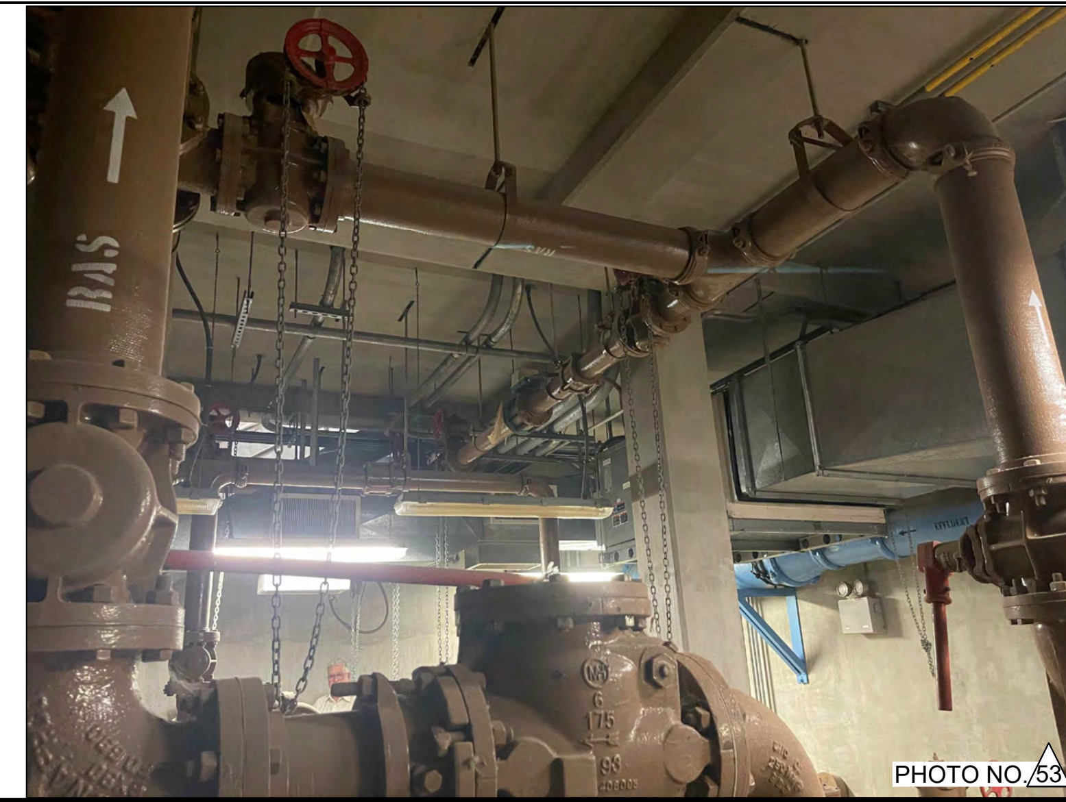
PHOTO OF THE OVERHEAD PIPELINES ON THE EAST SIDE OF EXISTING SLUDGE PUMP STATION LOWER FLOOR.
