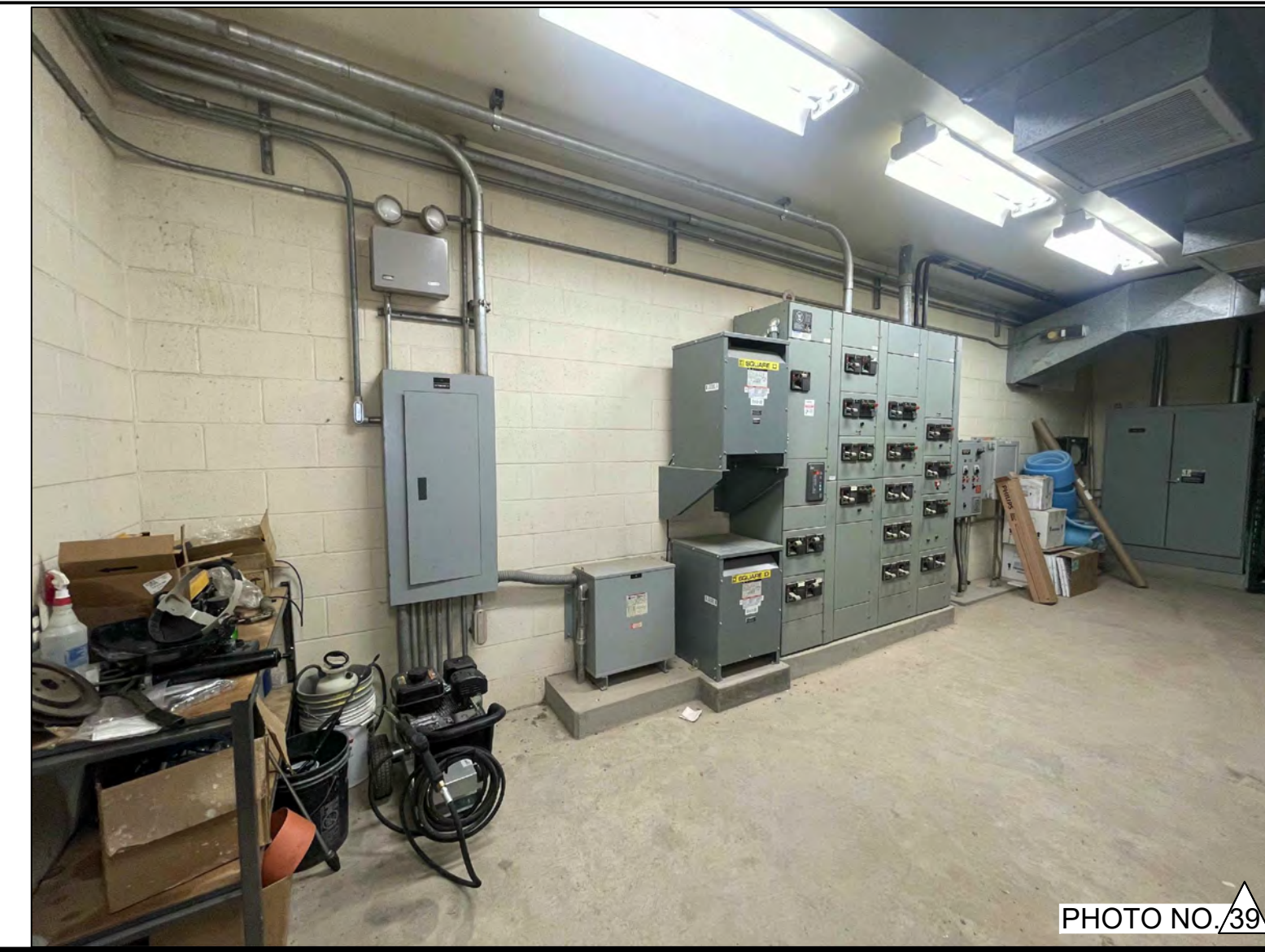
PHOTO OF THE SOUTH WALL OF EXISTING SLUDGE PUMP STATION UPPER FLOOR.
