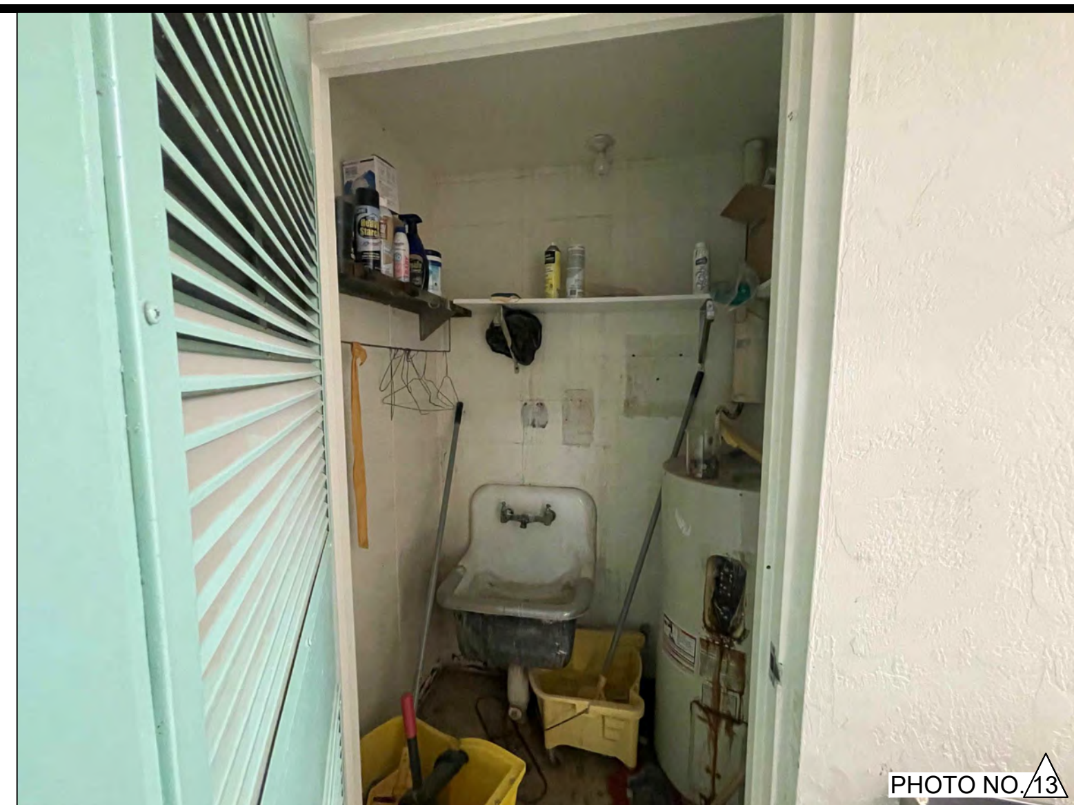
OPERATIONS BUILDING - PHOTO OF THE WEST WALL OF EXISTING BATHROOM. CLOSED AT THE EXISTING BATHROOM.
