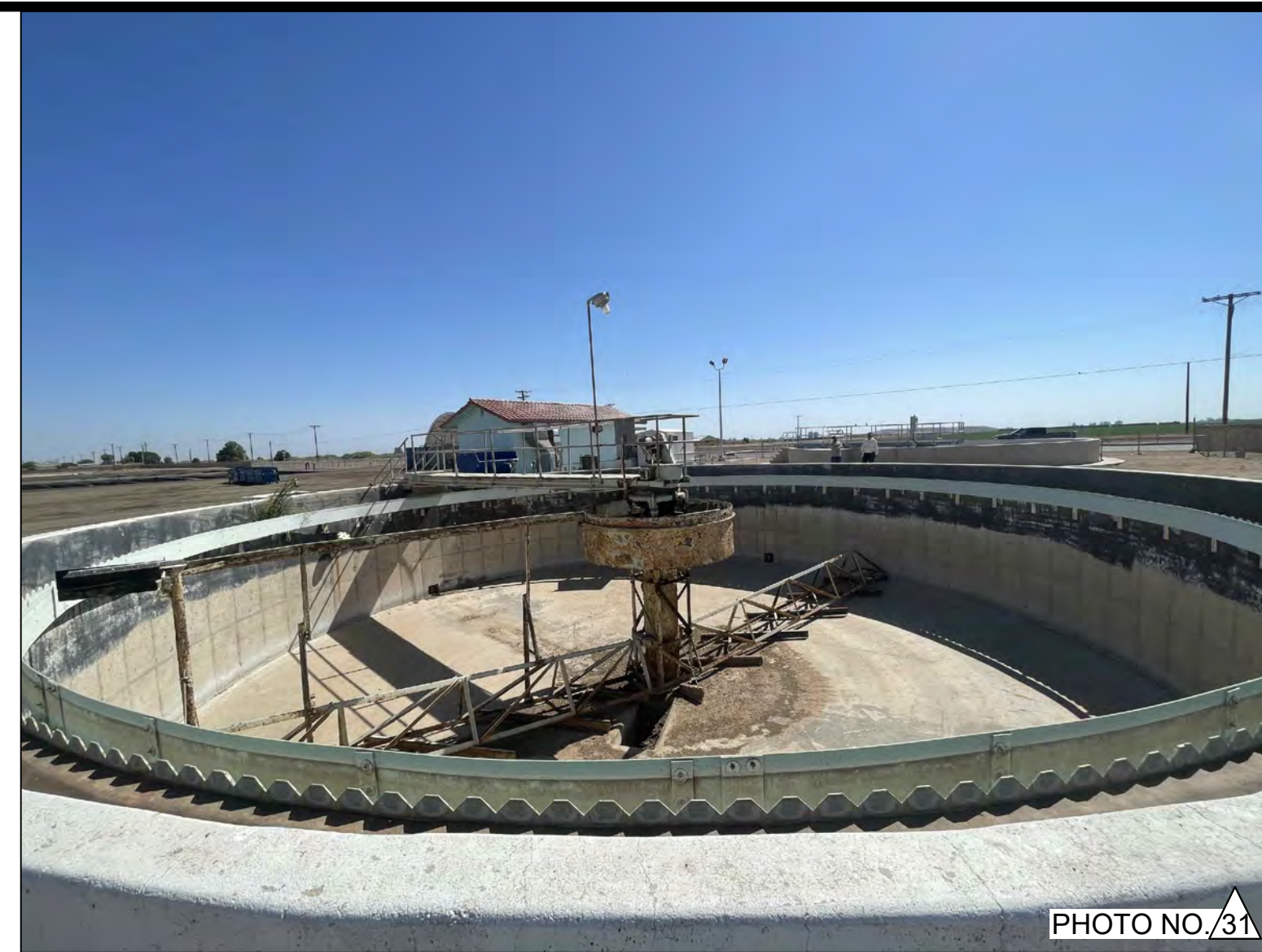
CLARIFIER NO. 1 - PHOTO OF THE SOUTHWEST SIDE OF CLARIFIER NO. 1 - TOP VIEW
